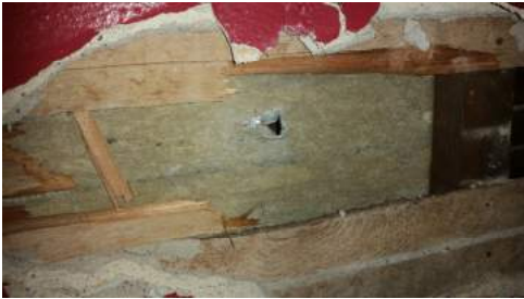
Duct Insulation, 1st Floor & Basement, 1 Duct Run to 2nd Floor
