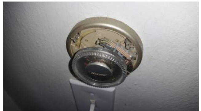
Mercury Thermostat, Room 8
