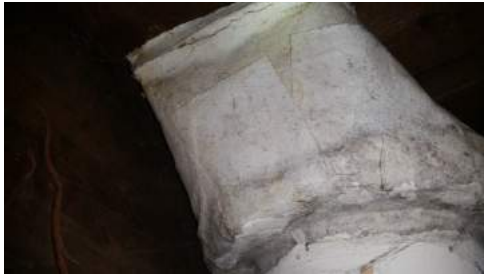
Duct Insulation, 1st Floor & Basement 3 Duct Runs to 2nd Floor
