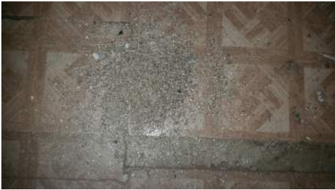
Vermiculite, 1st Floor Ceiling
