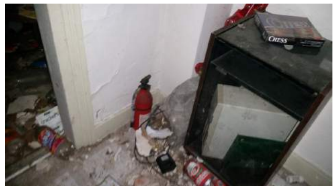
Fire Extinguisher, Room 8
