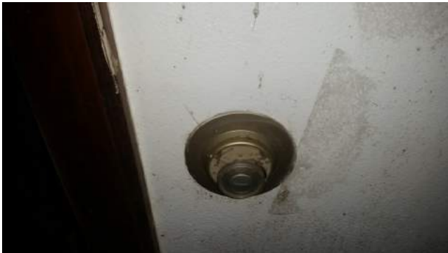
Mercury Thermostat, Room 2
