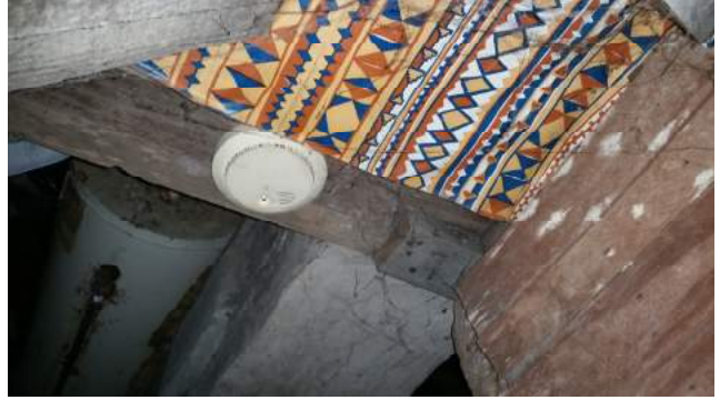
Smoke Detector, Room 10
