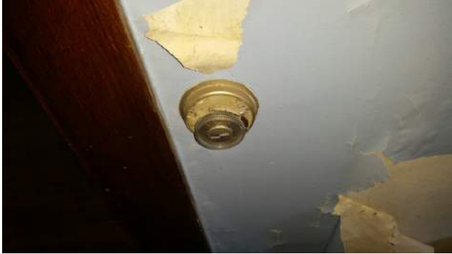
Mercury Thermostat, Room 1
