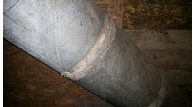
Duct Tape, Rooms 27 & 28
