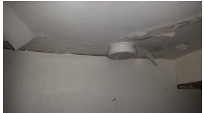
Smoke Detector, Room 15
