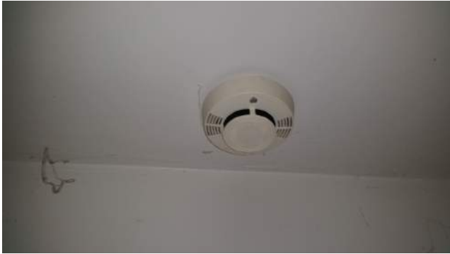
Smoke Detector, Room 8
