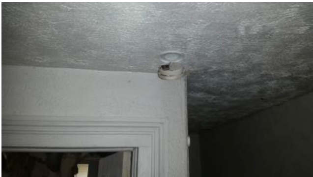
Smoke Detector, Room 24
