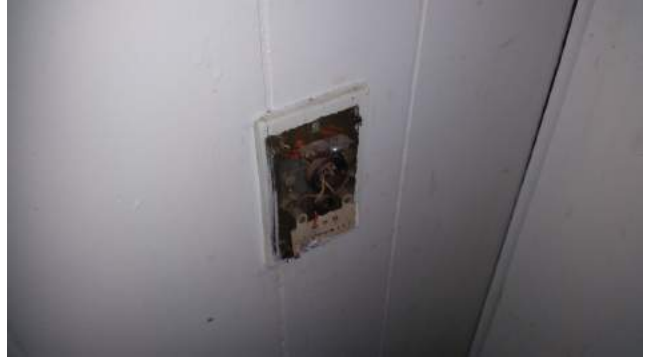
Mercury Thermostat, Room 8
