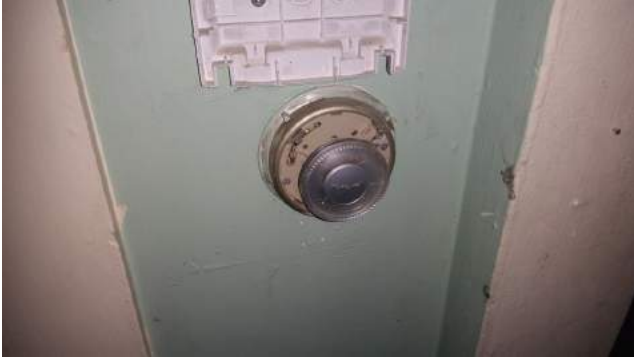
Mercury Thermostat, Room 2
