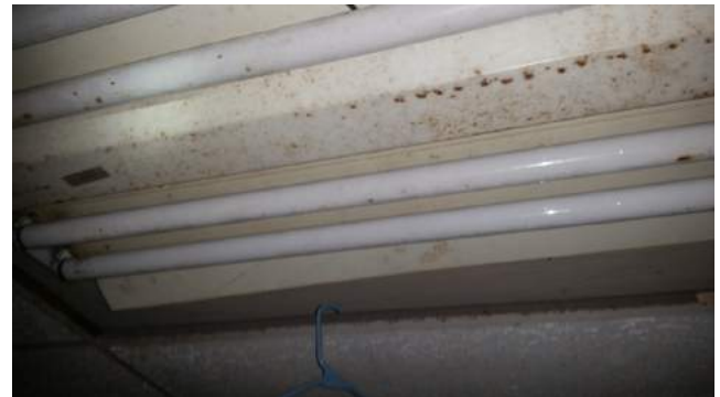
Fluorescent light tubes, greater than 4 ft, Room 3 & Room 27
