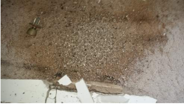
Vermiculite, 1st Floor Ceiling
