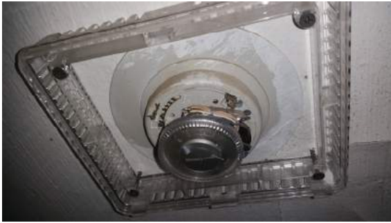
Mercury Thermostat, Room 1
