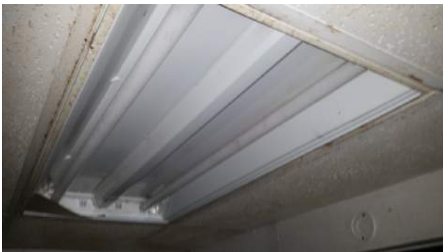
Fluorescent light tubes, greater than 4 ft, Room 2
